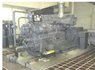
[自家発電設備]
